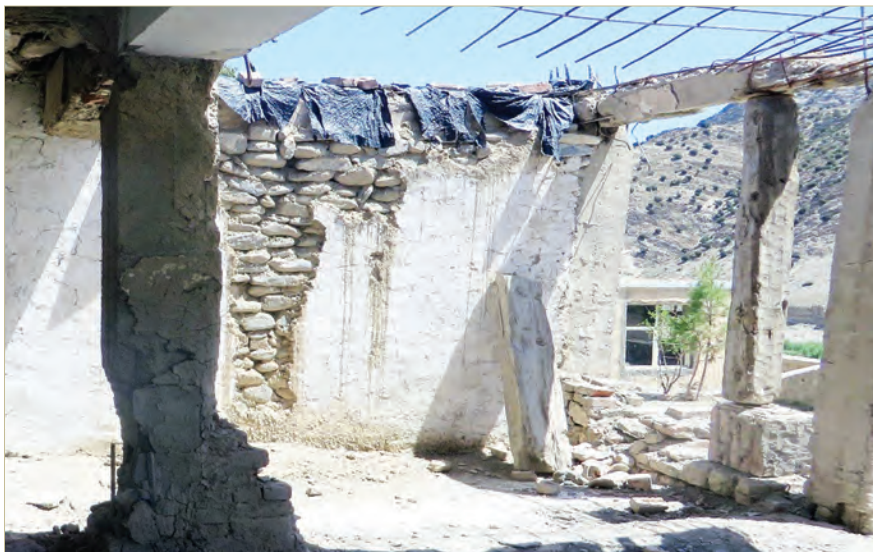
Construction at a Khowst Province health facility supported by USAID funds administered through a World Bank program. (SIGAR photo)
