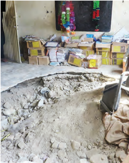
Serious foundation flaws at a school in Khowst Province. (SIGAR photo)
