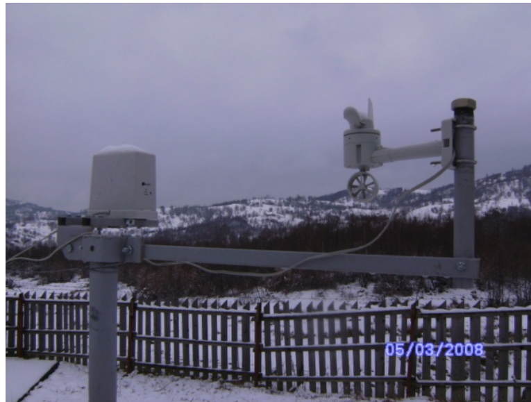
Figure 8: A part of the meteorological station installed at PLO4
