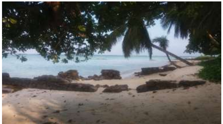
Picture 18: Degraded sea walls at Au Cap
