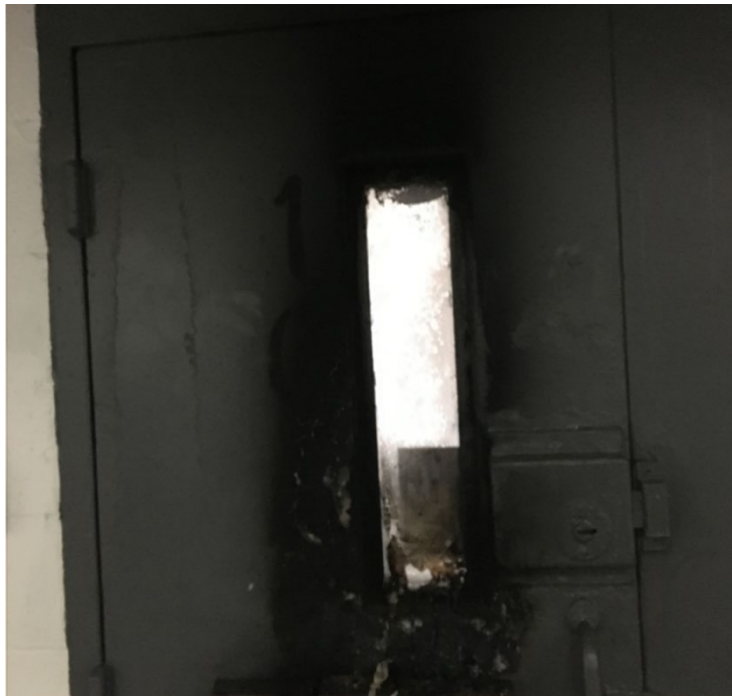
A cell door that had been burned from a fire inside the cell. The damage to the door made it so there was no visibility into the occupied housing cell.
