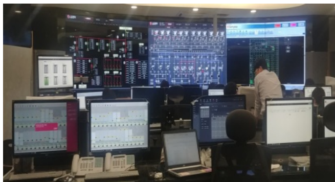
Figure 9 Medium control room
