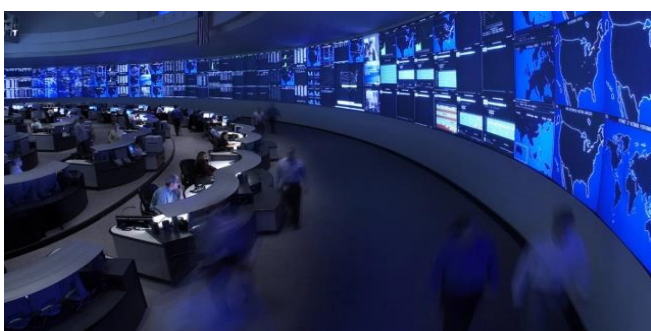
Figure 3 Telecommunications and network operation (Source: http://fortune.com/att-global-network-operations-center/ )
