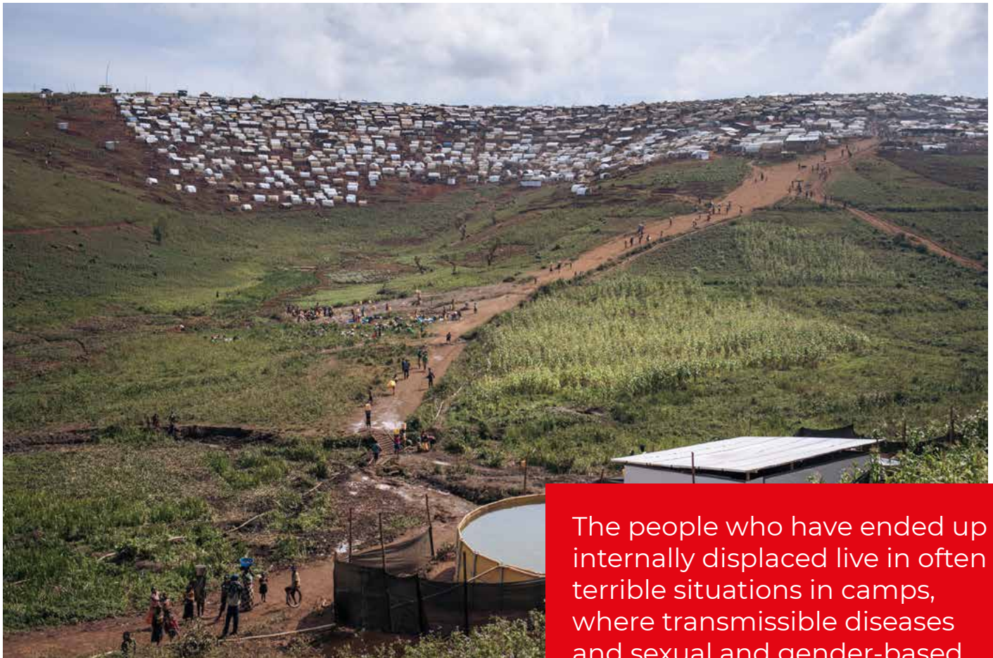
A view of the water, sanitation and hygiene facilities that MSF teams have installed in Rho displaced people's camp. Democratic Republic of Congo, December 2021. © Alexis Huguet
