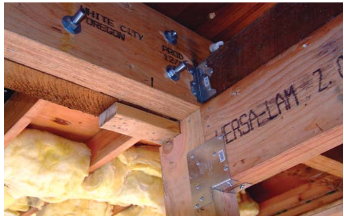
Napa, CA, Feb. 14, 2006 - A home is retrofitted with earthquake straps and bolts to prevent movement in the event of an earthquake (Photo credit: FEMA).
