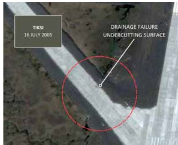
Figure 80: Tiksi south taxiway erosion Google Earth 07/16/2005
