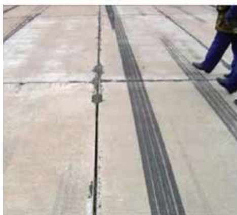
Figure 25: Prefabricated concrete slabs (left) and welded joint (right). Adapted from Damage to Russian Arctic airfields and their supporting infrastructures poses a direct threat to Russia’s ability to project power and capitalize on economic opportunities in the region. Airfield surfaces and foundations, drainage features, and supporting facilities like fuel storage depots are all critical to the safe and effective functioning of an airfield. These airfield features are also all at risk of damage due to the unstable ground created by thawing permafrost. https://www.researchgate.net/publication/347228859_Reconstruction_of_the_Technical_Condition_of_Concrete_Airfield_Pavements_with_the_Use_of_Prefabricated_Slab_Technology
