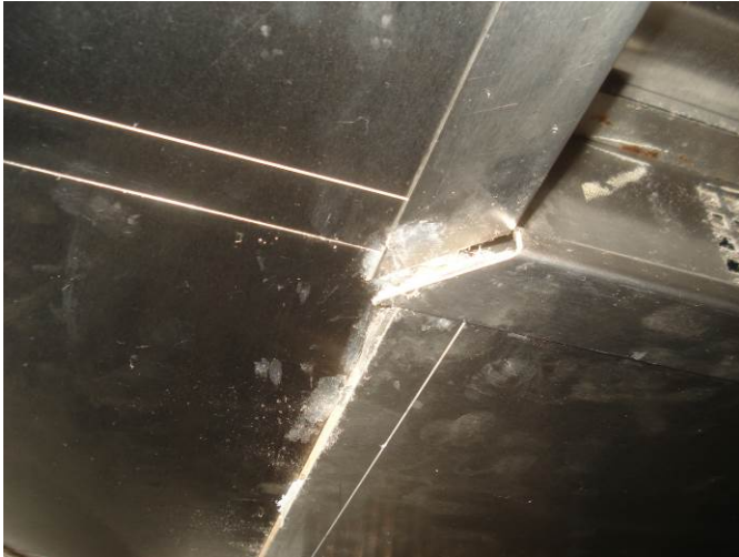
17. Repair ceiling where a portion appears to be coming loose
