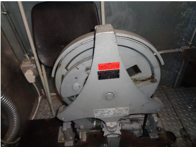
7. Dover Governor should be replaced.
