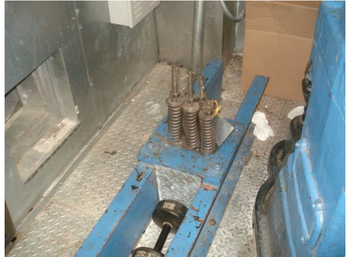
18. Remove dumbbells from machine room. By code, only elevator equipment is allowed in machine room.
