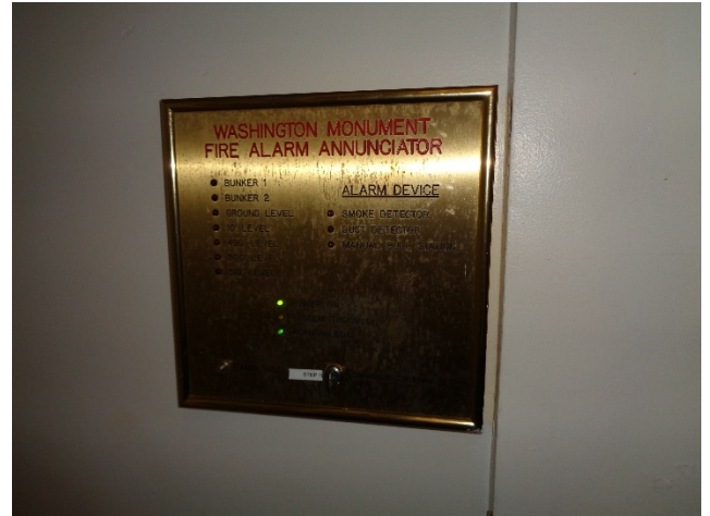
2. A new fire alarm panel should be provided.
