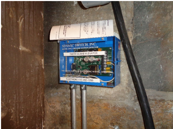
11. Existing seismic monitor to be retained.
