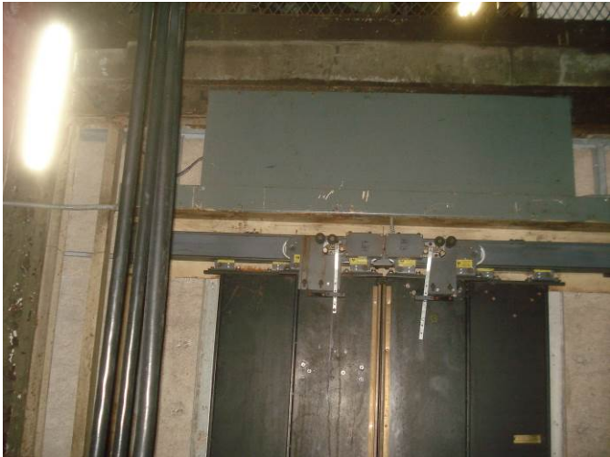
8. Replace missing dust covers
