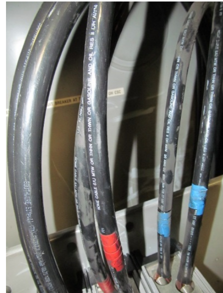
Figure 8: Mismatched Conductor Sizes (250 MCM vs 2/O) in Siemens Circuit Breaker Panel
