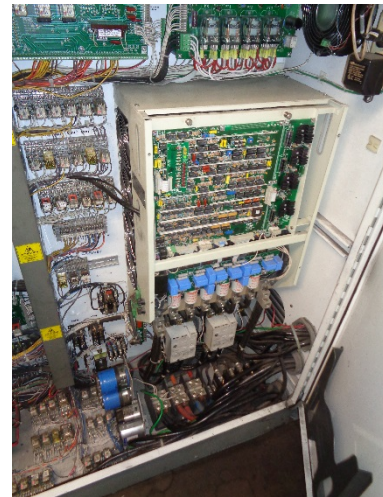
8. MCE controls need to be replaced.
