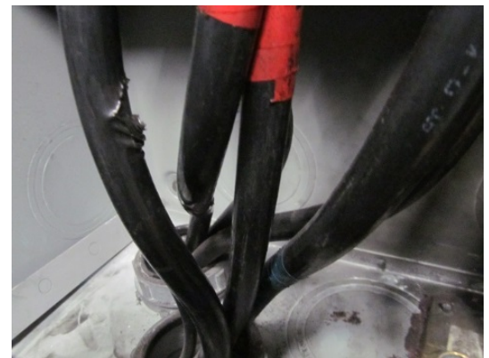
Figure 7: Peeling Skin on Cable (Left Conductor) in Siemens Circuit Breaker Panel
