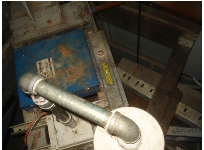
24. All wiring on car top should be protected
