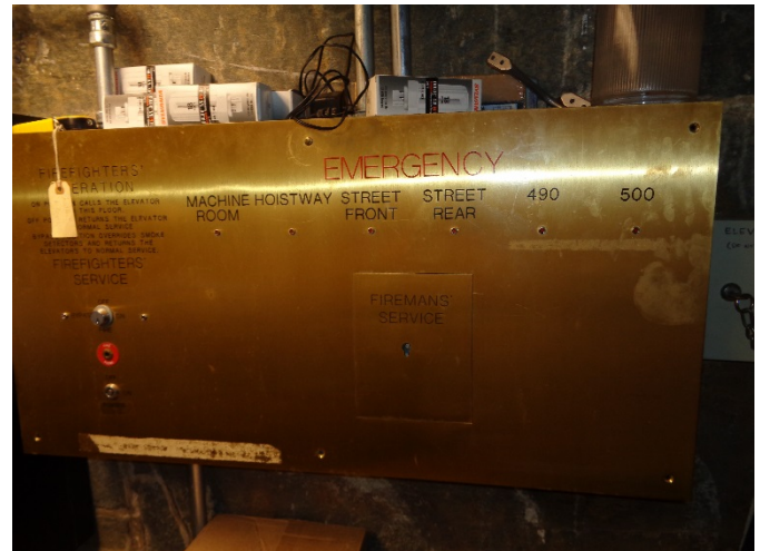
12. Existing fire control panel to be replaced.
