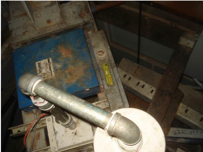
7. Cartop light needs to be operational
