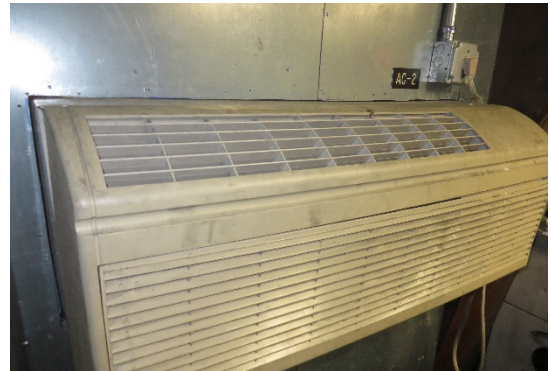
Figure 6: Interior Trane PTAC Unit (AC-2) in Poor to Fair Condition
