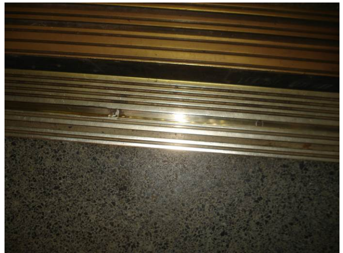
12. Car sill is worn and requires replacement
