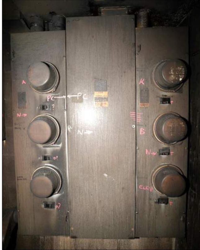
Figure 27 - Service entrance metering gear. (August 15, 2023, TJB)
