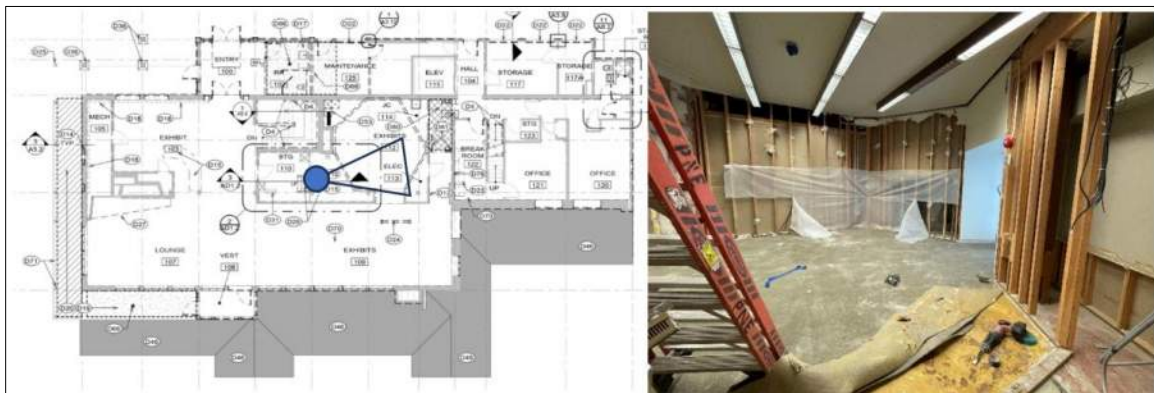
Figure 11- Exposed wood structure near the "Theater" Area (Main level, facing east, April 25, 2023)
