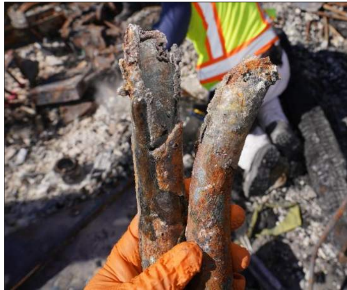
Figure 31 - Arced conduits from the main level (Fed from XB). (August 16, 2023, TJB)
