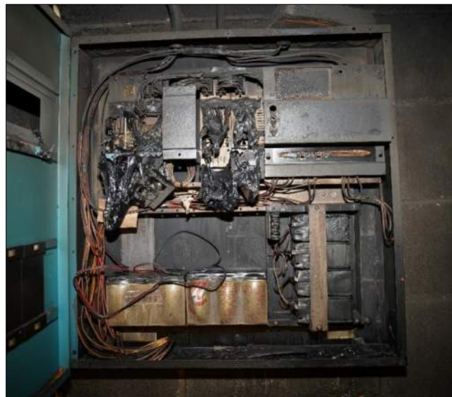
Figure 28 - Pyrotronics System-3 Fire Alarm Panel. (August 15, 2023, TJB)
