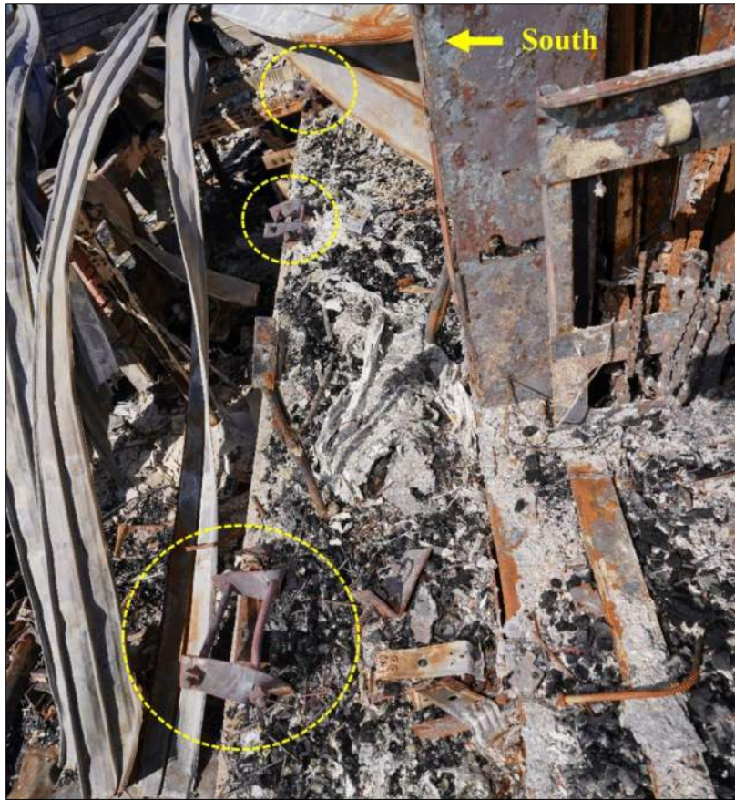
Figure 15 - Column brackets bent toward the southern exterior of the structure. (August 16, 2023, TJB)
