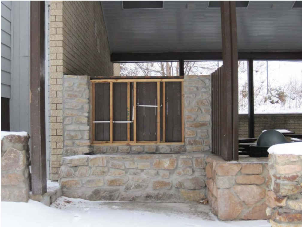
Figure 1 - Filling station under construction. Note proximity of table in adjacent concession food area
