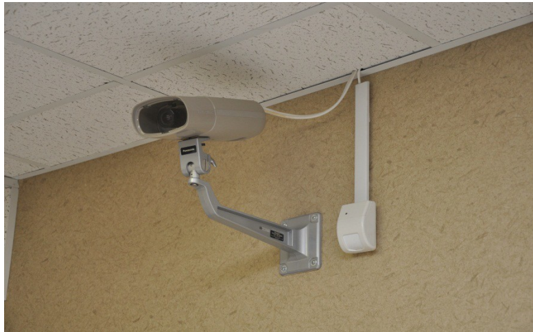
Figure 4-9 Example of a VMD camera
