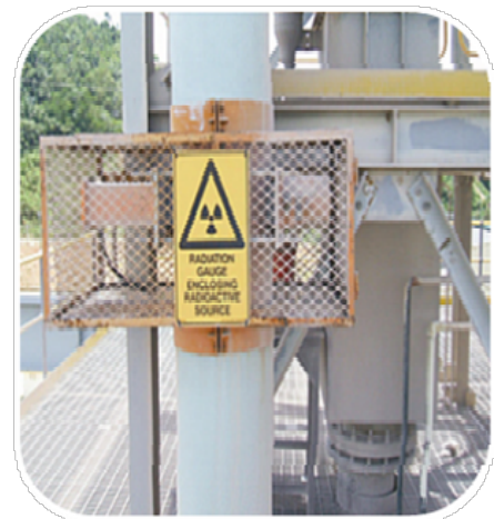
Figure D-2 Example of a physical barrier surrounding a fixed gauge
