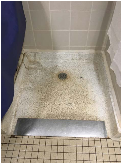
18 Grime/mold in detainee shower area
