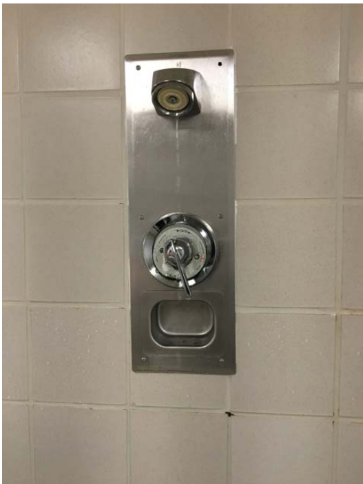
22 Leaking shower head
