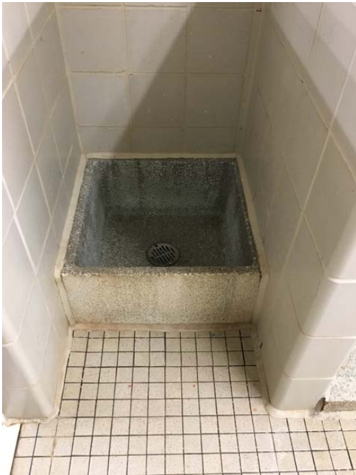
16 Mold/grime in detainee washing area
