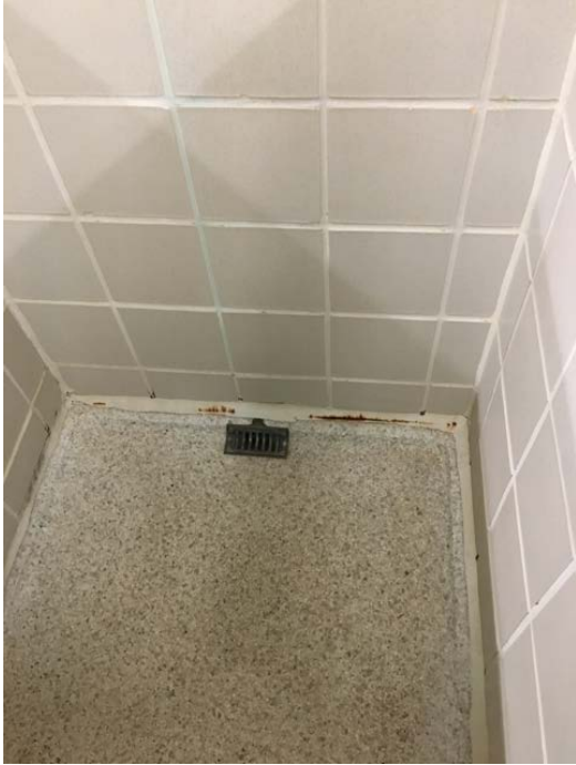
19 Grime/mold in detainee shower area
