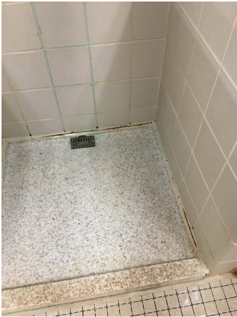
20 Grime/mold in detainee shower area
