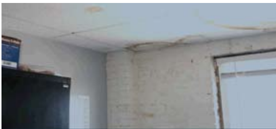
This March 2006 photograph illustrates an interior office in the ANT/WPB Building, Sector Southeastern New England, and demonstrates the deteriorating conditions of the building.
