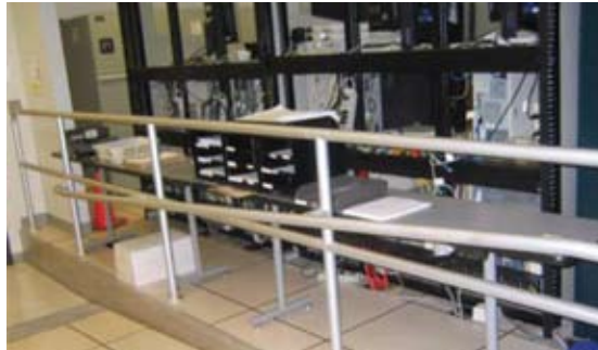
Computer Room Printout Desk. This illustrates how printouts are not segregated and restricted, but are commonly placed on a table near the entrance to the computer room. Nearby, USCIS places daily backup tapes for couriers.
