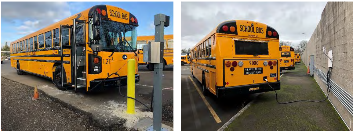
Figure 6. Pedestal (Reynolds School District) and wall mount (Beaverton School District) chargers at Oregon electric school bus pilots
