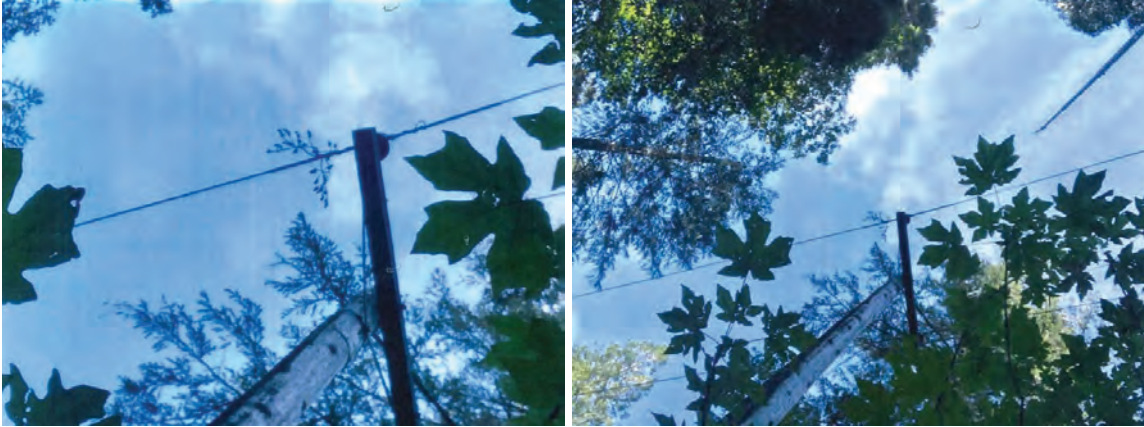
Figures 2 and 3: In Chico, Butte County, a tree branch landed on a PG&E conductor.
