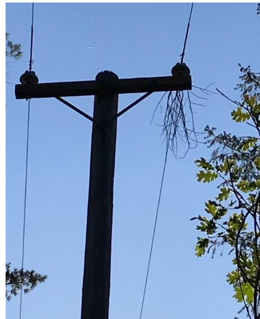
Figure 2 – Vegetation Debris Near 98 Gamble Rd, Oroville
