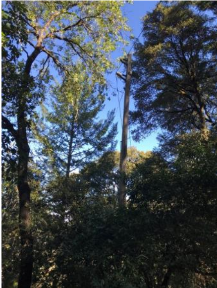
Figure 13: Image of Vegetation Related Damage in Santa Clara County - Broken and Floating Primary Insulator
