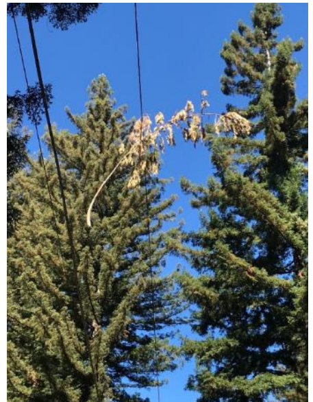
Figure 18: Image of Vegetation Hazard in Santa Clara County - Tree Branch Blown into Conductor
