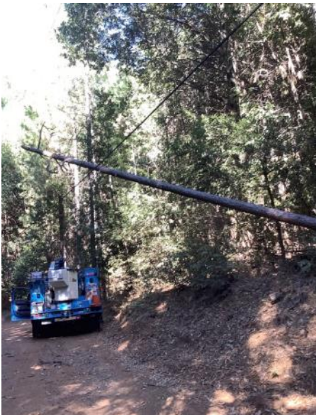
Figure 16: Image of Vegetation Hazard in Butte County – Dead Pine Tree Fell on Conductor
