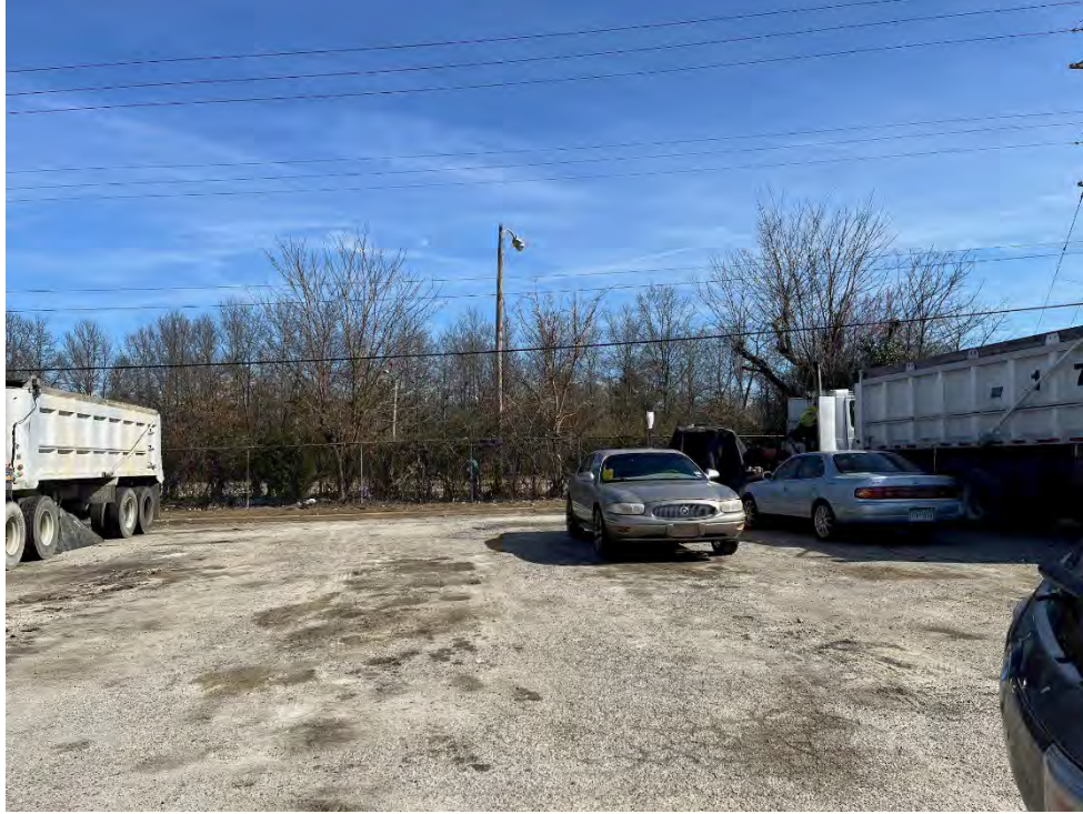
Photograph # 31 – Representative portion of asphalt parking area in central area of site, immediately north of commercial buildings (3/1/2024)
