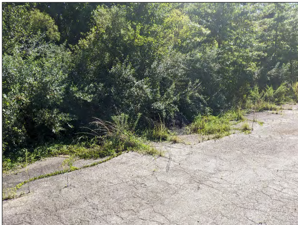
Photograph 6. View of push piles along the southwestern border of the APE, facing east.
