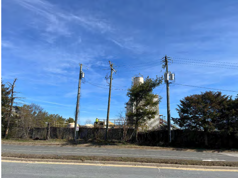
Photograph # 23 – Power poles and transformers adjacent to Vulcan materials plant; “Non PCB” labeling visible from ground. Also visible in Photo # 21. (3/1/2024)
