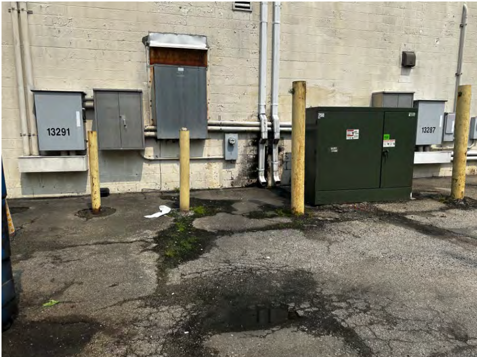
Photograph # 12 - Utility connections for onsite buildings (typical) (7/13/2023)
