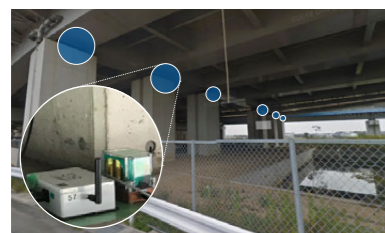
The installation of acceleration sensors and wireless devices enables the remote, real-time detection of abnormalities in bridge beams and columns during disasters and in other situations.
