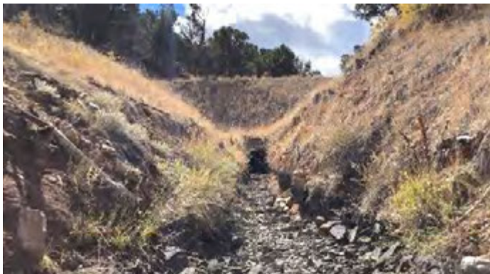
Outlet of the Gould Canal lower tunnel and beginning of canal section 2, proposed for lining.
