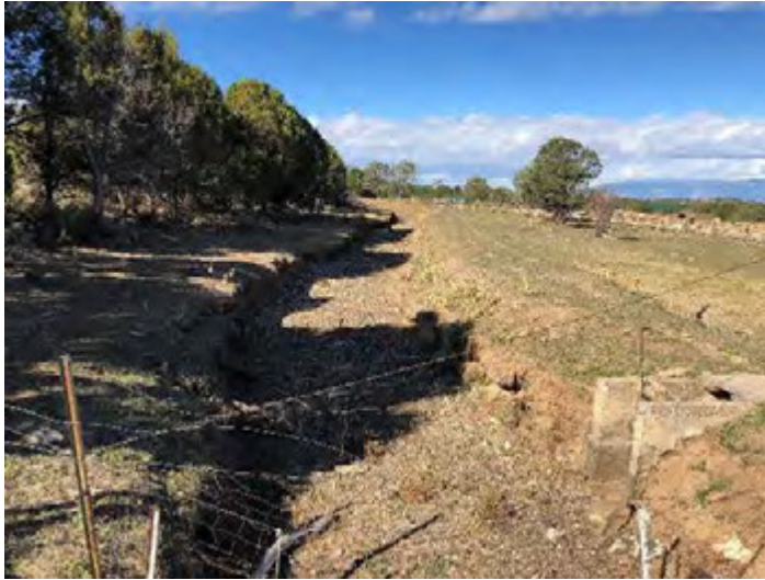
Gould Canal section 4, proposed for lining.
