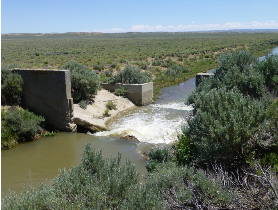
Figure D-3. Upstream side of the drop structure nearest to the headworks of the Big Sandy Feeder Canal.
