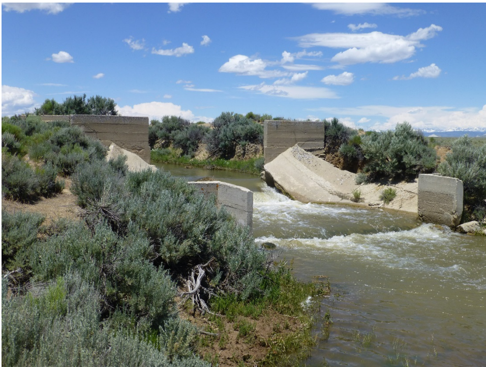
Figure D-4. Downstream side of the drop structure nearest to the headworks of the Big Sandy Feeder Canal.
