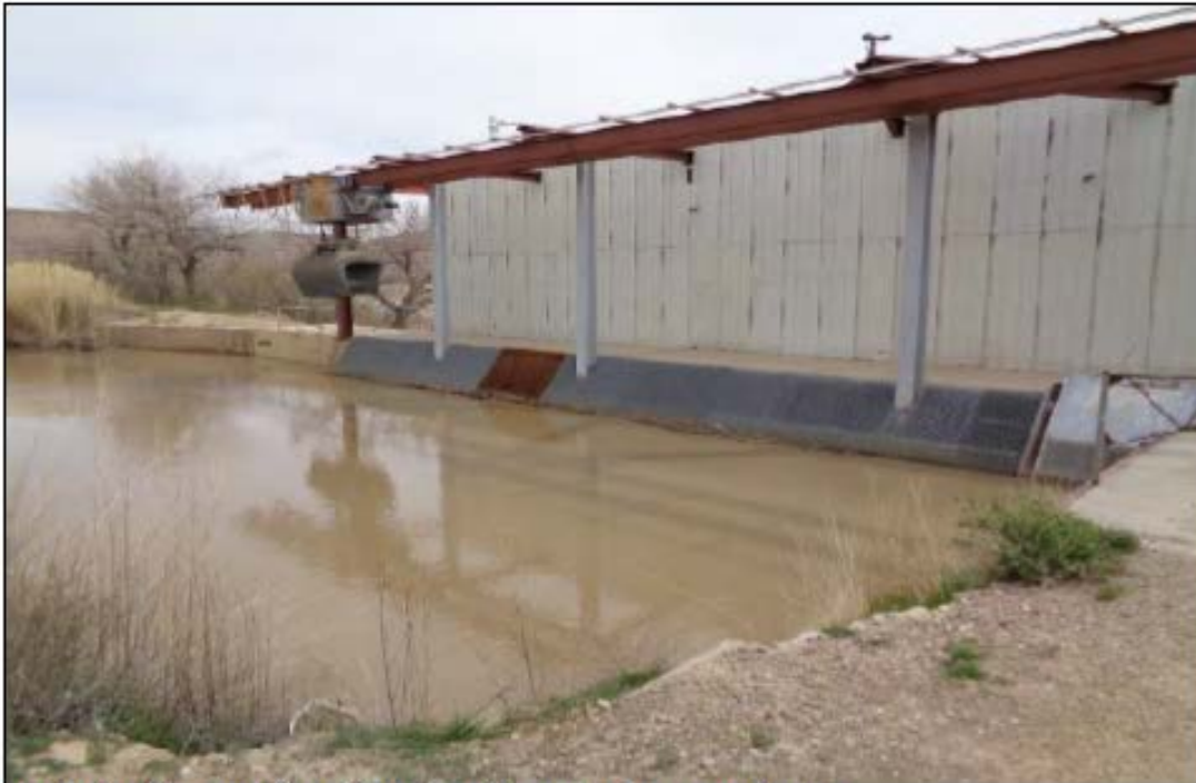
Photo 3. View northeast showing Thayn hydropower plant
