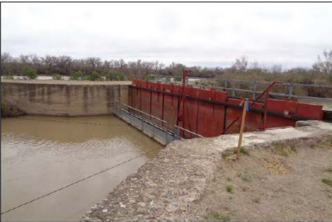
Photo 6. View southeast showing 8-gate structure to be replaced (southcentral of Action Area #1)
