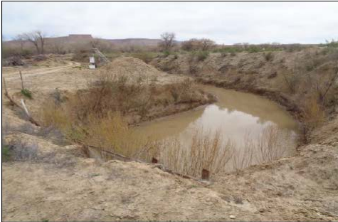
Photo 7. View south of inverted siphon outlet that will be replaced as part of the proposed project
