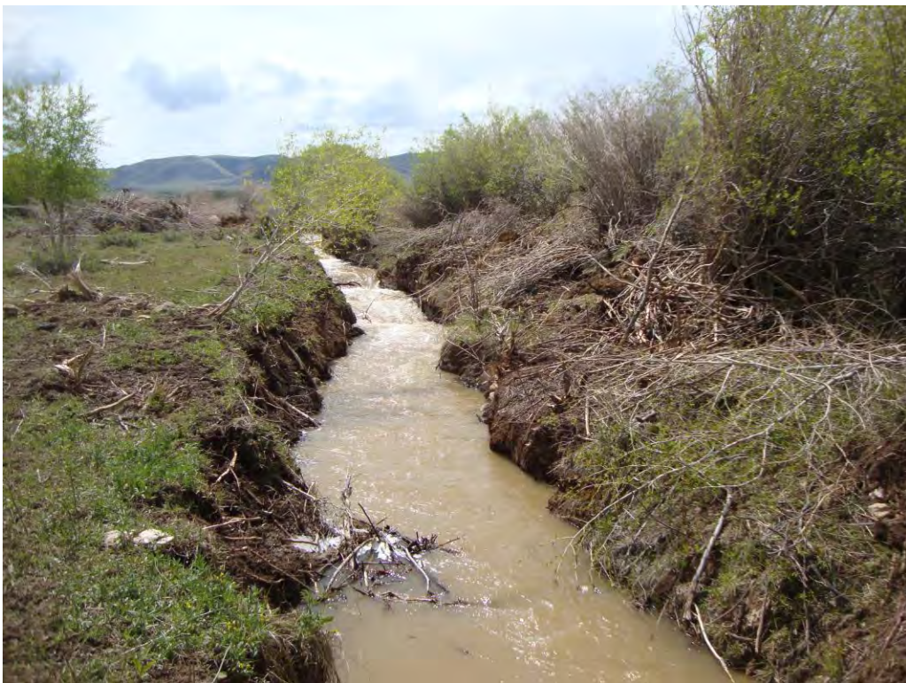
Photo 3. A section of the Antelope Lateral that is north of and parallels SR 43 where regular maintenance has occurred, looking west.
