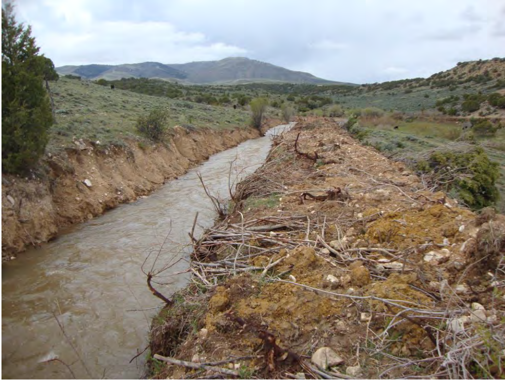
Photo 2. Typical section of the Antelope Lateral where regular maintenance has occurred, looking west along a section that will be abandoned and filled in.
