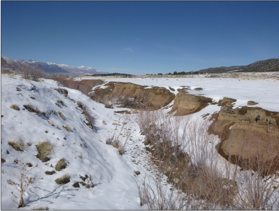
Figure 3-3 Round Valley Creek Ditch
