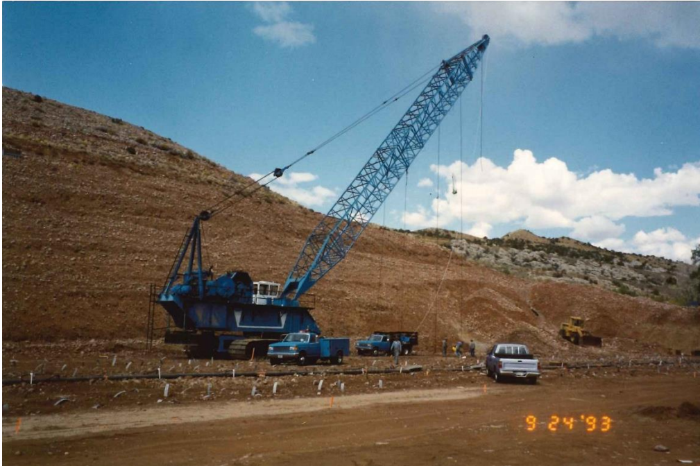
Figure 0.11 The Thumper Crane, Project photograph CN-325-418-340, Photograph by Tom McCarl on 9/24/1993.
