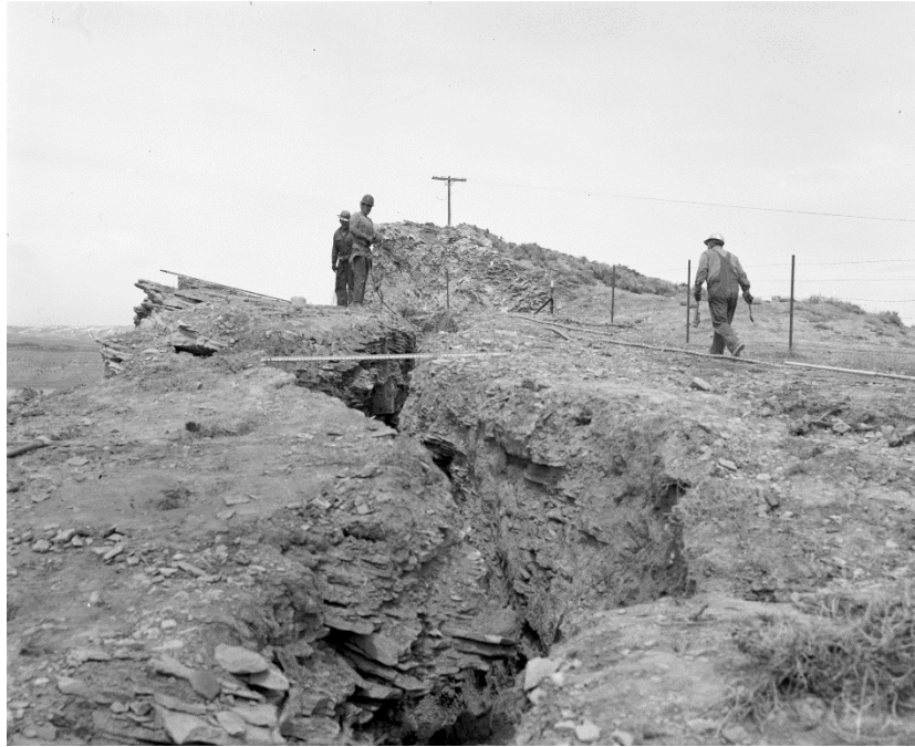
Figure 0.9 View of crack in the left abutment of dam. Workmen are drilling holes for blasting. Project photograph P325-418-1239, photograph by R. H. Felter, April 1966.
