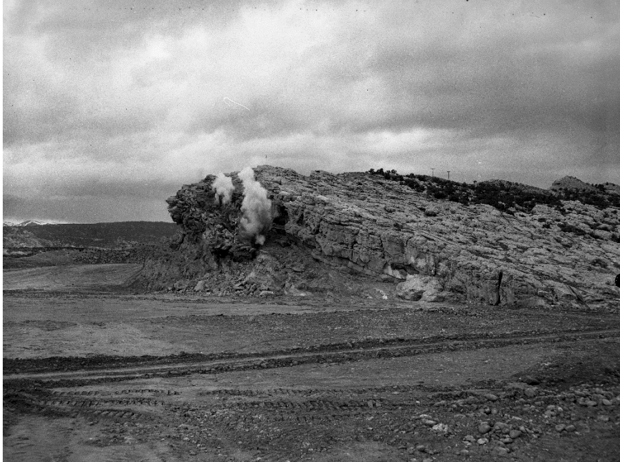
Figure 0.3 Photo is taken during first blasting operation. Looking toward left abutment. Project photograph P325-418-0264, Photograph by Elmer S. Davis, 3/26/60.
