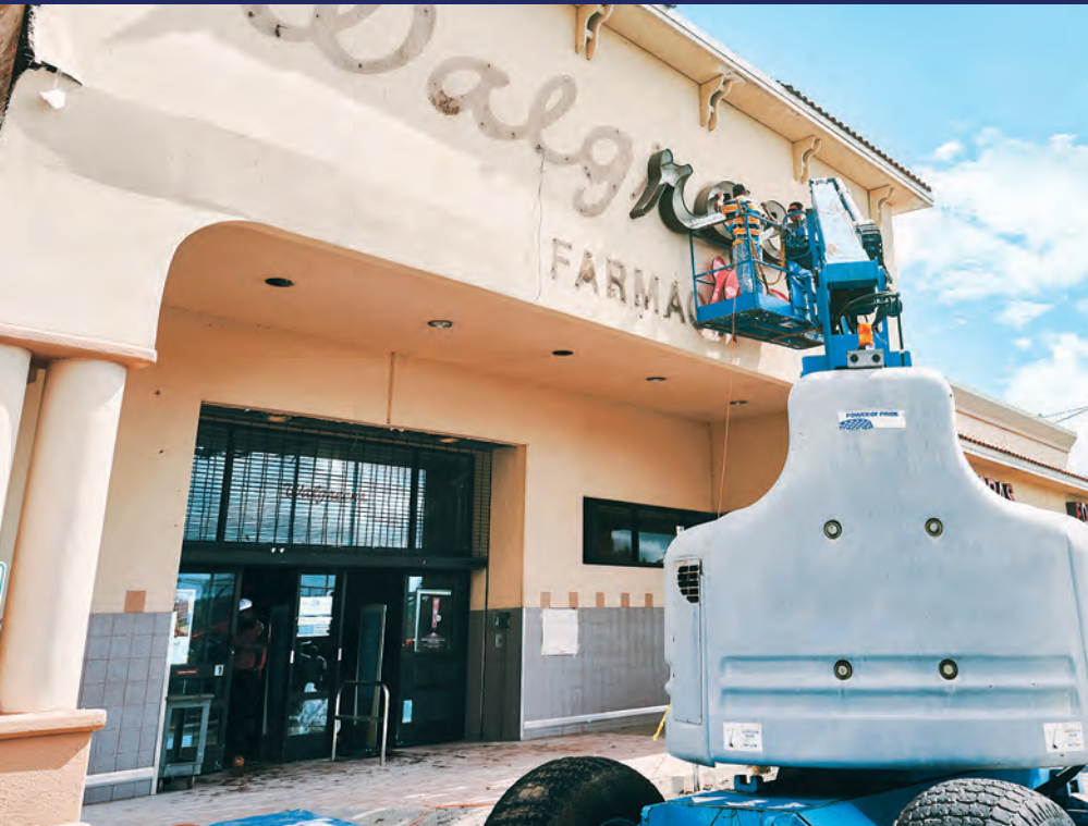
A Walgreens store in Puerto Rico is repaired after suffering damages in Hurricane Maria.
