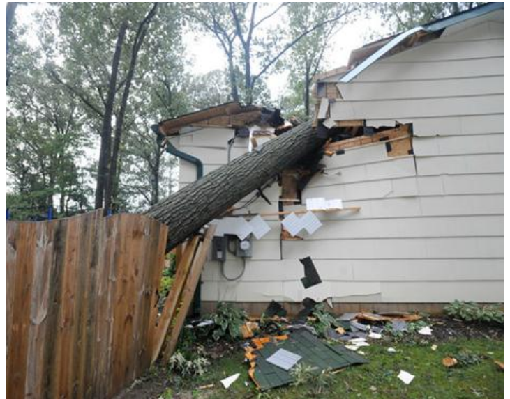
Storm Damage in Severna Park, MD
