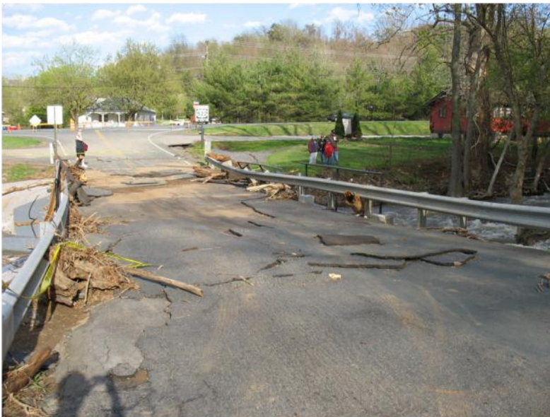
Water overtopped this bridge on Criser Road in Front Royal. The bridge was closed for nearly a week while repairs were made
