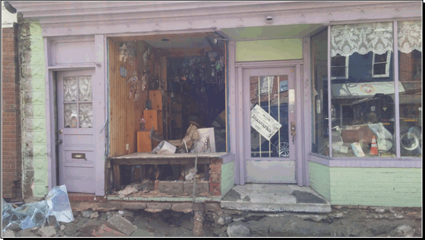
The power of the water rushing downhill ripped out the sloped brick sidewalk in front of buildings on 8200 Block of Main Street in Ellicott City, Maryland. Credit: NWS Survey Team
