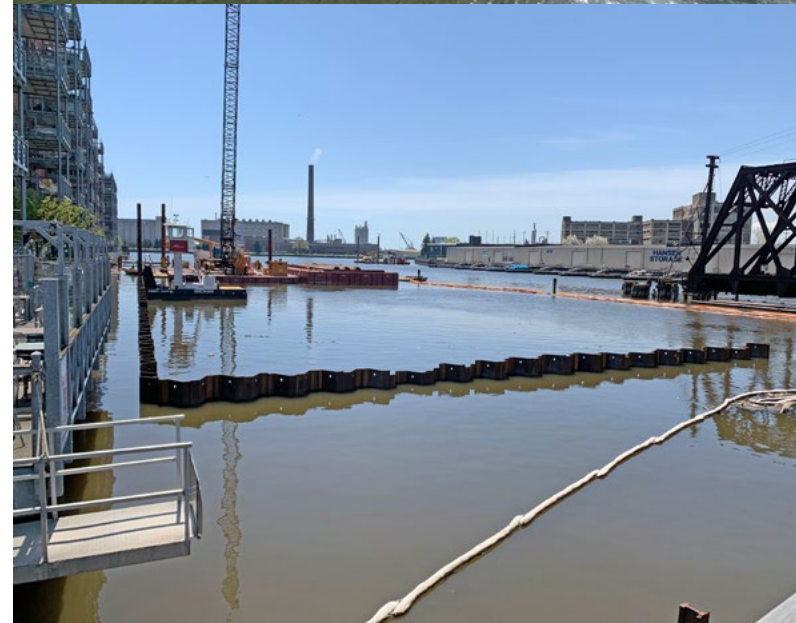
Top: Engineered cap material being installed on the river bottom. Bottom: Installing steel sheet pile
