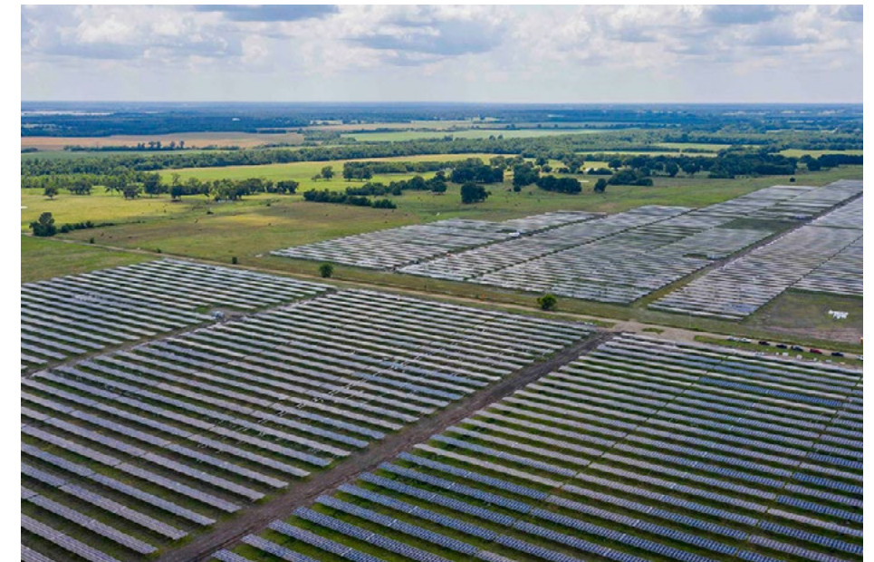
Samson I Solar Energy Center, part of our WEC Infrastructure portfolio
