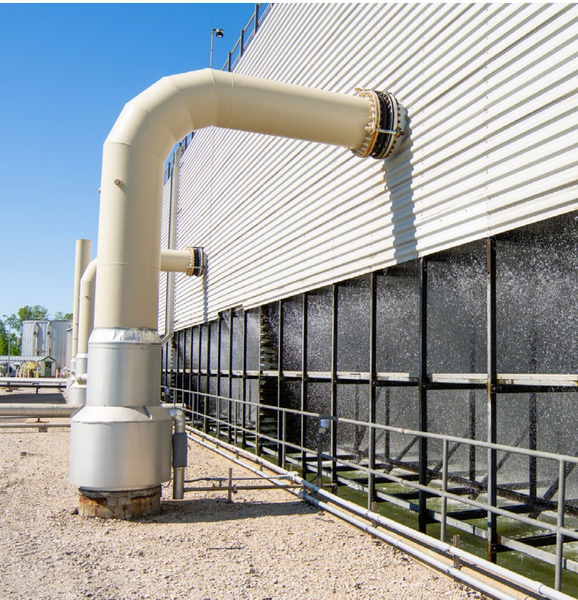
Fox Energy Center cooling tower
