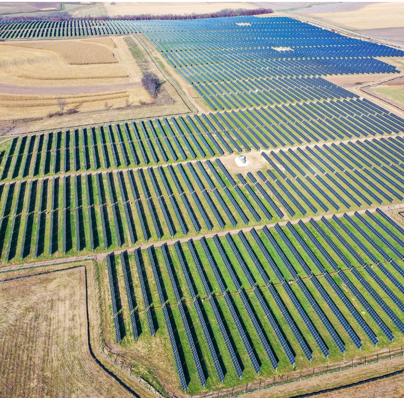
Badger Hollow Solar Park I
