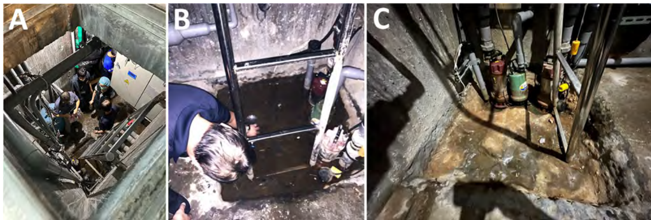
Figure 2. Basement mechanical area in an investigation of a fatal case of Naegleria fowleri primary amebic meningoencephalitis from indoor surfing center, Taiwan, 2023. A) The opening to the basement with ladder visible to right of opening; B) stagnant water beneath the basement ladder; C) depression under basement ladder after water was drained.
