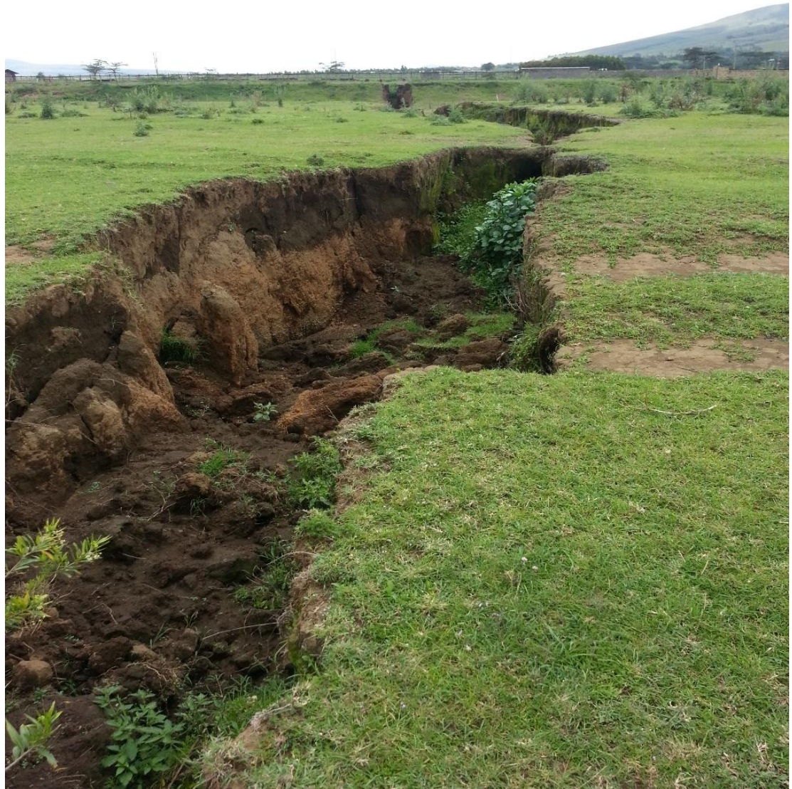
Figure 7: The Maai Mahiu-Naivasha C88 Road fissure
