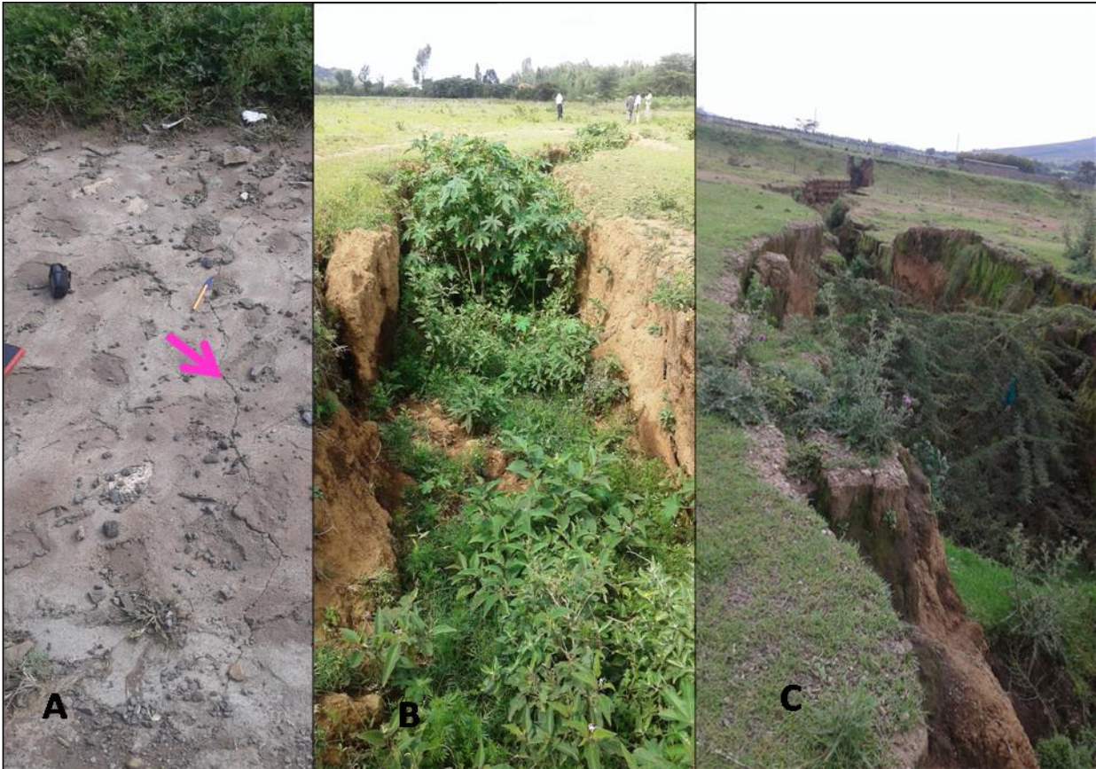
Figure 18: A) Fresh developing crack on the road pavement; B) Fissure developed during the period when the road was cut off; and C) Wide fissure formed northwest of the research project area.
