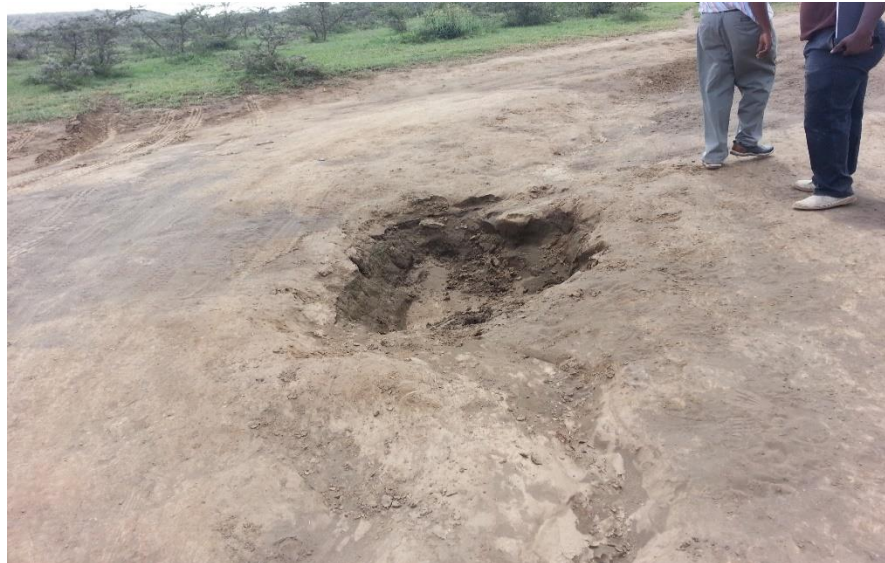
Figure 6: Other developing fissure on Maai Mahiu-Narok road
