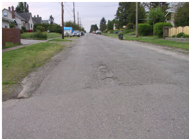
A poorly defined street edge and deteriorated pavement on S Monroe St.
