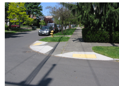
Curb ramps at every intersection provide safe and comfortable access for people with disabilities.
