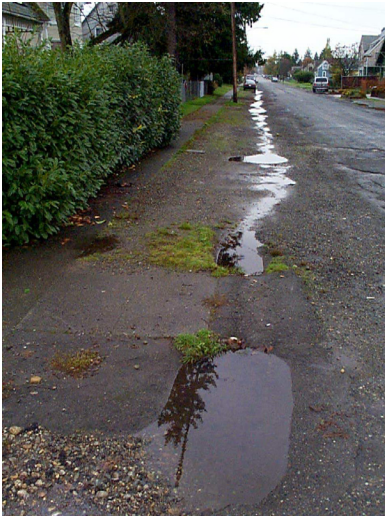
Poor drainage along S Junett St., an oilmat street.
