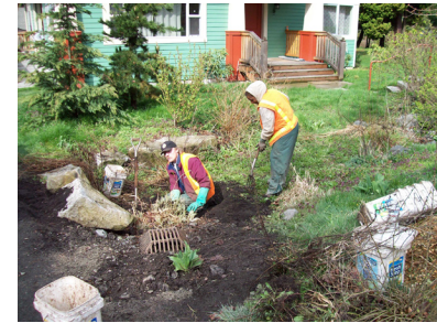
Natural drainage systems require periodic maintenance, a major consideration in the design and installation of these facilities.
