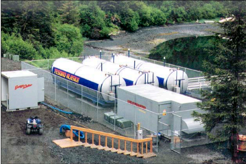
This is an upgraded tank farm with secondary containment.
