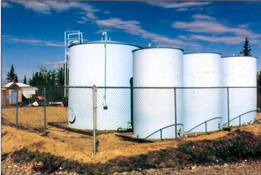
Fuel tank farm.
