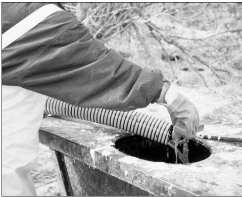
Flush-haul operators may be exposed to raw sewage when emptying the tank.
