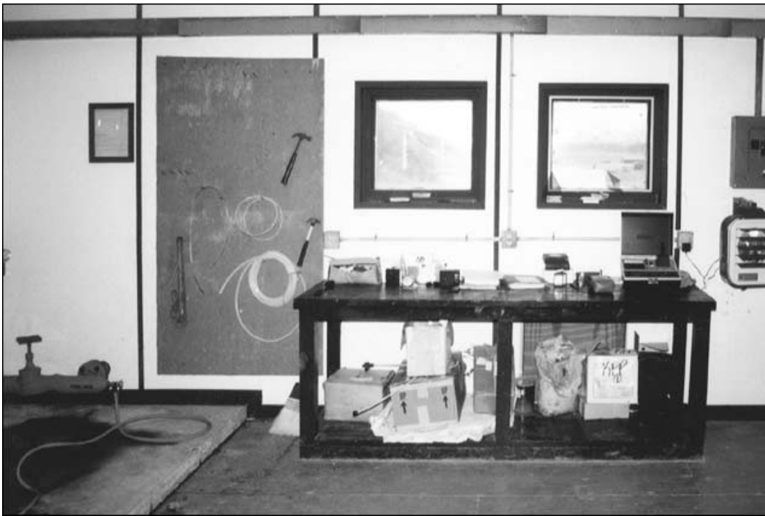
A clean water treatment plant is often a good sign of the operator's quality of work.
