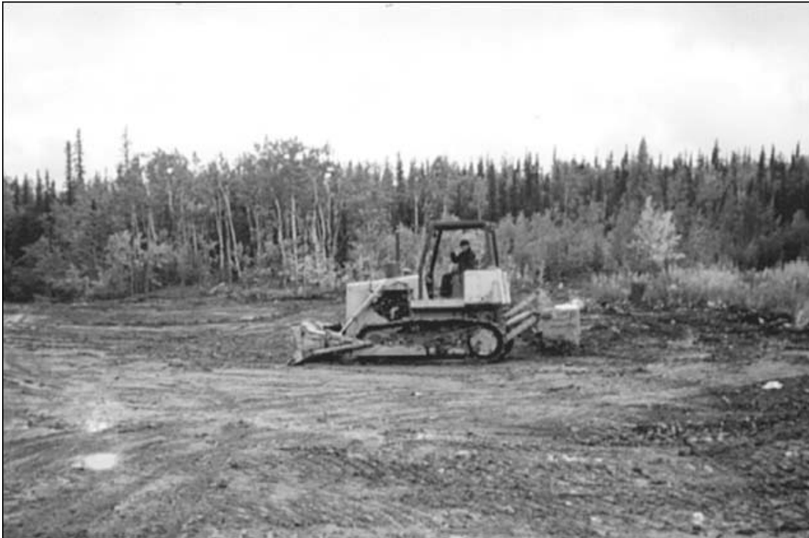
A bulldozer is being used to consolidate, compact and cover waste at the landfill.
