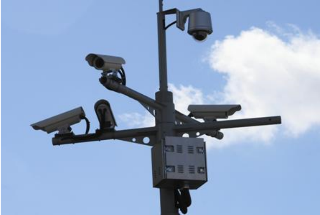
Figure 1.2: An Exemplary Installation of Cameras for an ITS Application
