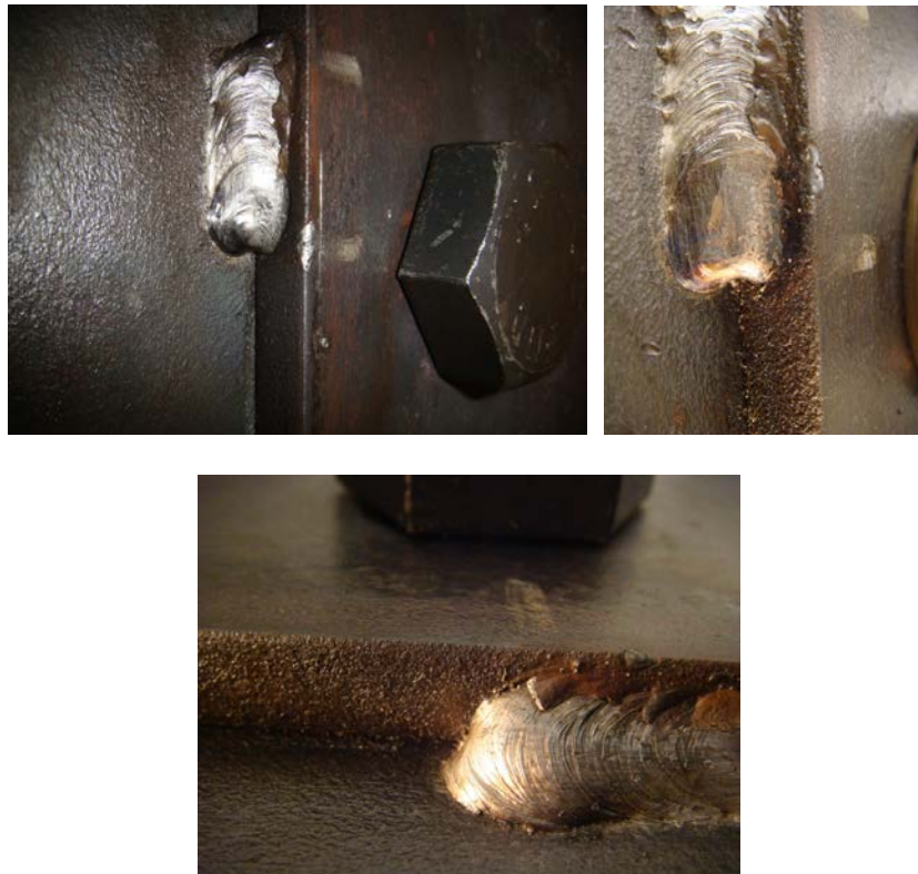
Fig C-23: Specimen TW-2LM-12-2 Tack Weld Cracks
