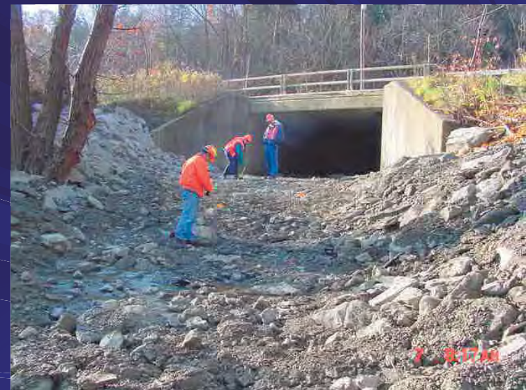
Rte. 36 / Rock Spring Creek Repairs 11/03 Re-built stone channel downstream to re-establish profile
