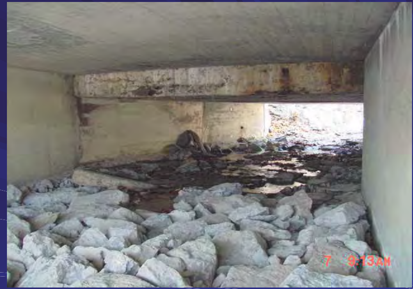
Rte. 36 / Rock Spring Creek Repairs 11/03 Grout under footings, grout-filled bags and heavy stone to fill
