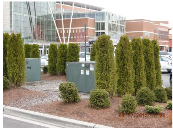
Figure 18-48: Using evergreen landscaping to screen utilities
