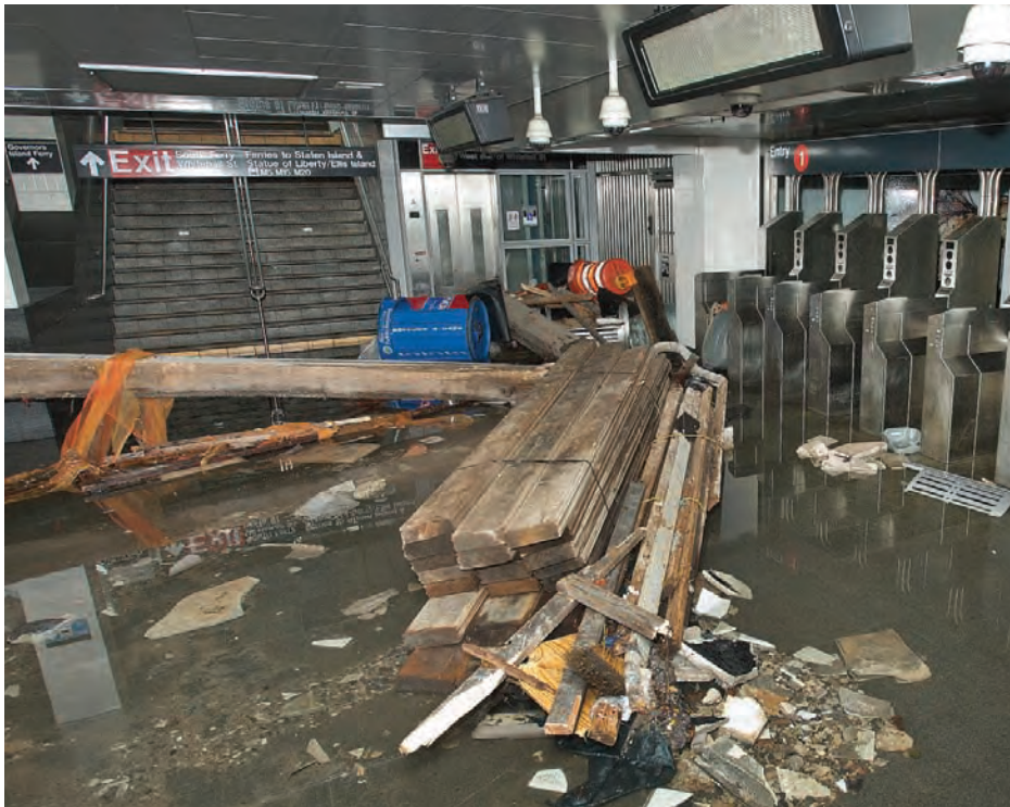
The South Ferry Station in Lower Manhattan was flooded to the mezzanine level.
