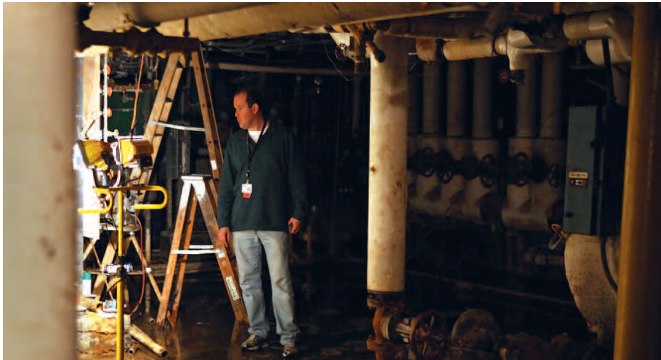
Coney Island Hospital staff survey the flood-damaged basement after Sandy.
