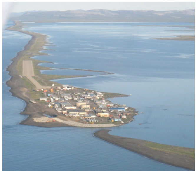
Rock revetment project, Kivalina, Alaska. Source: Millie Hawley, Manager Kivalina Environmental Program
