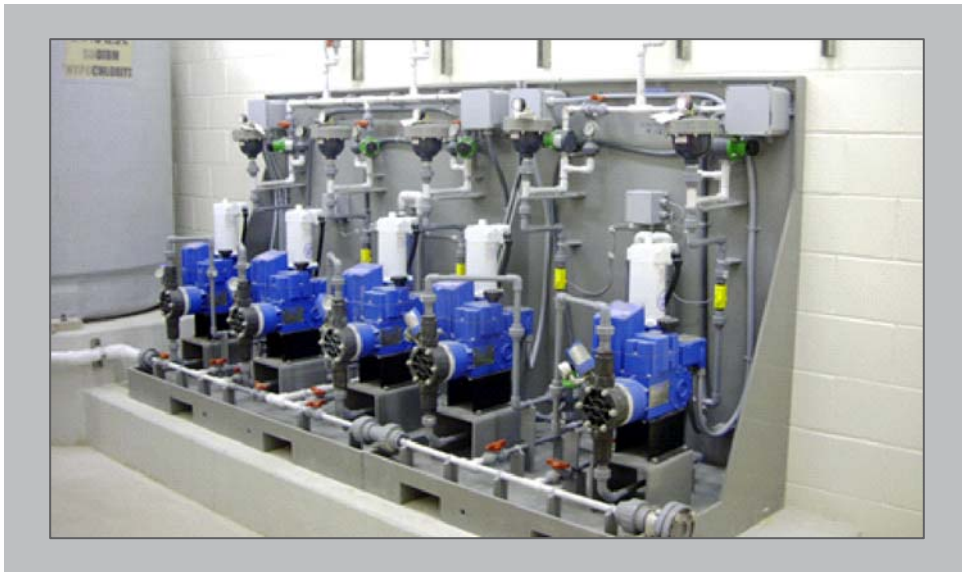
Figure D-9. Chemical Production Pumps
