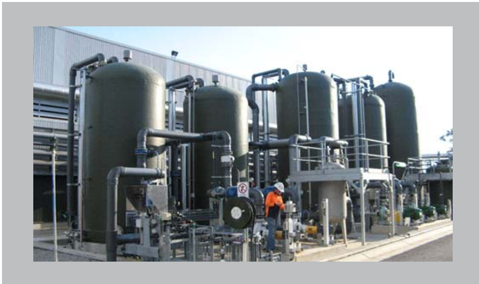
Figure D-3. Chemical Storage Tanks
