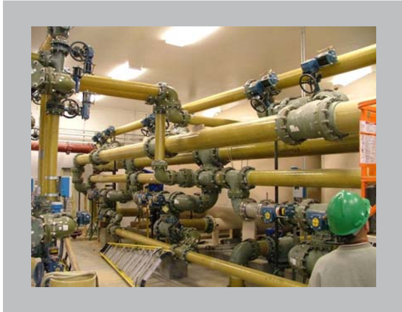
Figure D-8. Chemical Processing Piping
