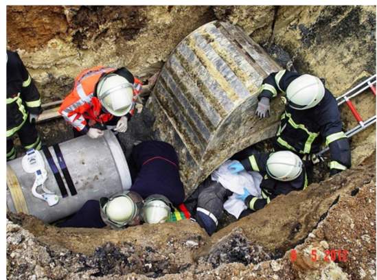
Figure 3. Worker pinned by detached bucket [8]
