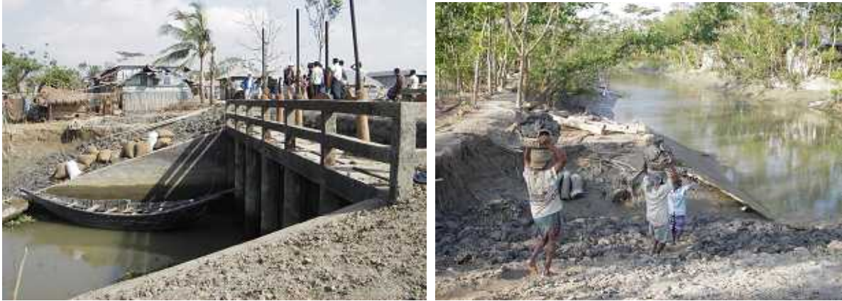
Fig. 1-3-3A Bridge damaged by the storm surge and the Rehabilitation work
