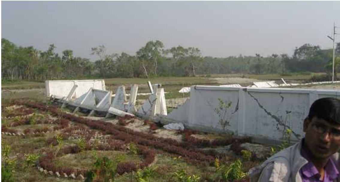
Fig. 4.20 Concrete walls around the botanical garden. Walls parallel to shoreline were all collapsed while some walls perpendicular to the shoreline survived.
