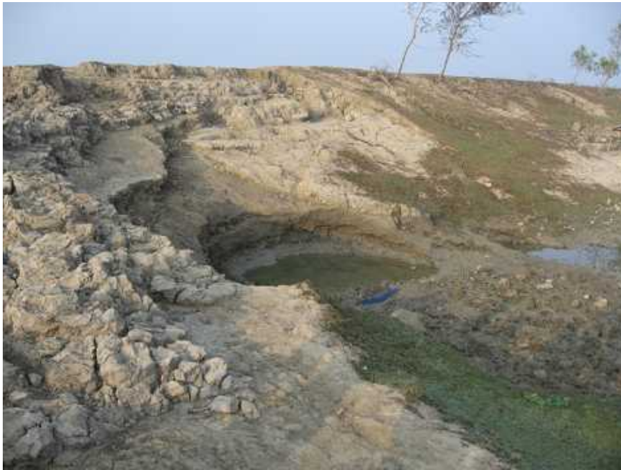
Fig. 4.13 Scour behind the crest of embankment in West Kuakata
