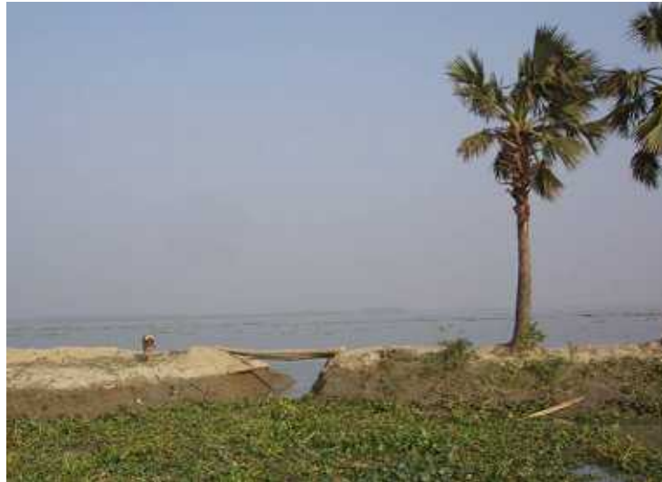
Photo 2.10 Broken river bank in Southkhali
