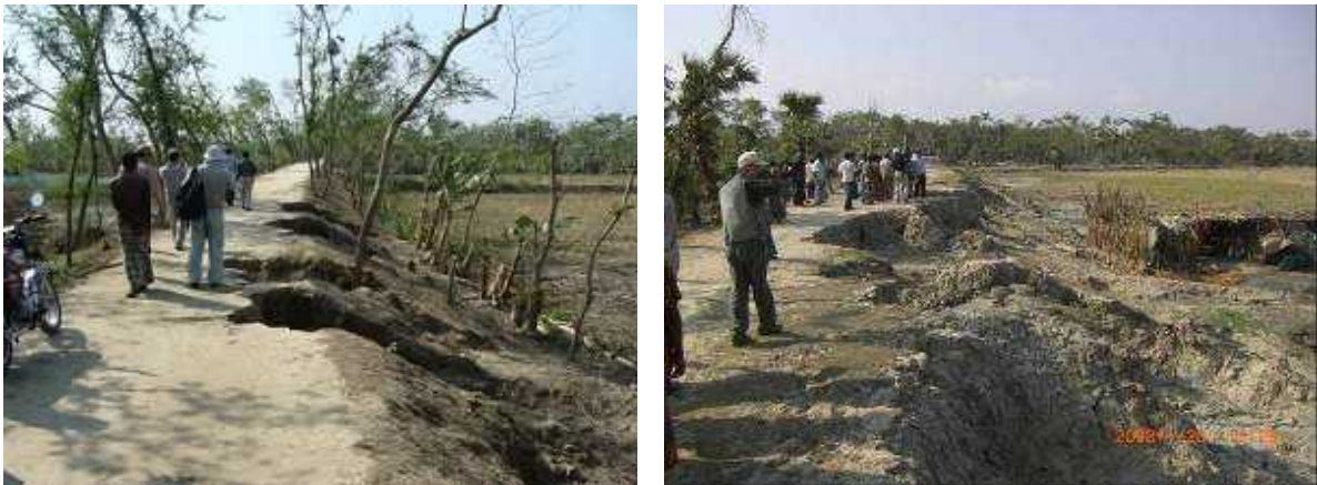
Fig. 1-3-4 Inner banks damaged by the storm surge at Sapleza, Mathbaria
