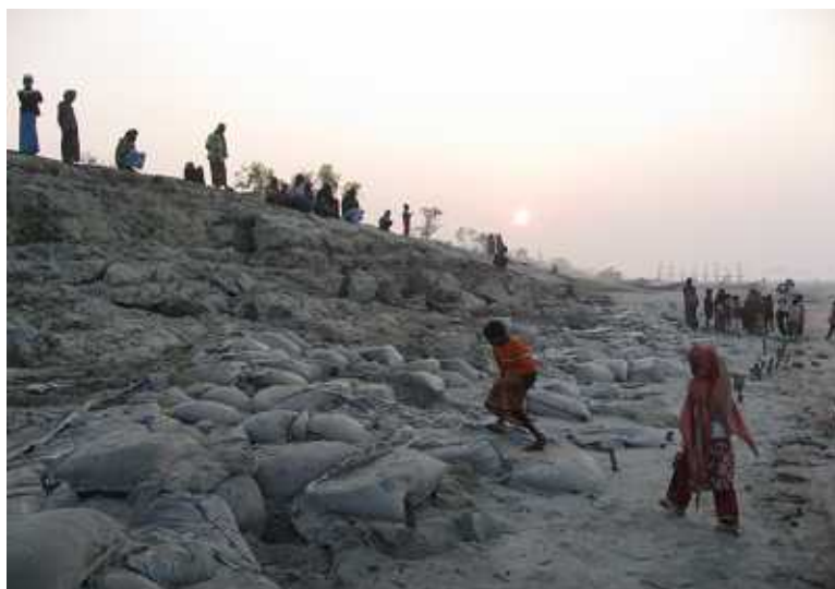
Fig. 4.12 Front side of the embankment with sandbags in West Kuakata
