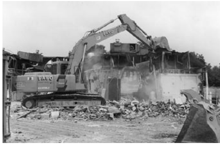
The demolition of Park Forest Plaza mall. Photo courtesy Village of Park Forest.
