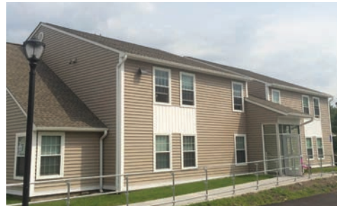
Left: West Broadway Villas deteriorated over time.
