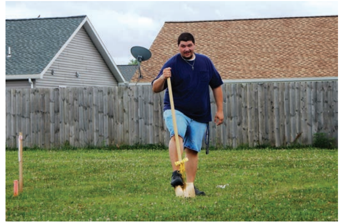
Coburn breaks ground to begin construction on his home, built through USDA's self-help housing program.
