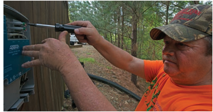
A worker fine-tunes the installation of broadband equipment to bring high-speed Internet service to members of the Choctaw Nation in Oklahoma.
