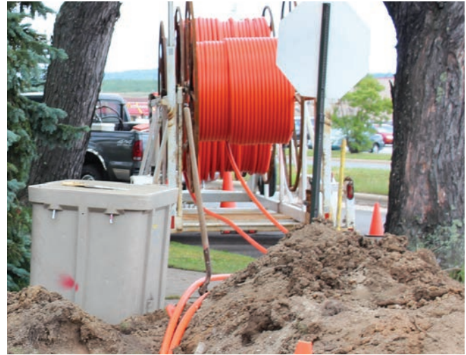
Giant spools of fiber optic cables used for the USDA-financed Minnesota Iron Range high-speed broadband network.
