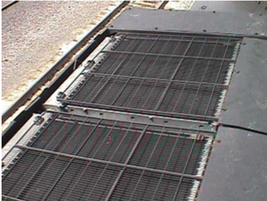
Photograph 6-11. Cooling Grid (Do Not Walk On)
