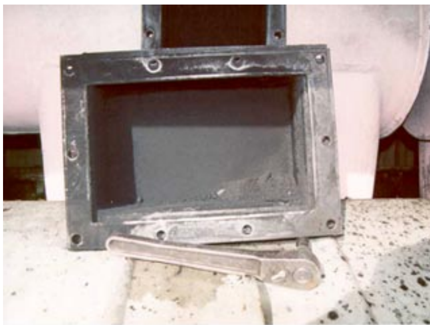
Photograph 5-7. Clean-Out Trap (Note Carbon Lower-Left Corner)
