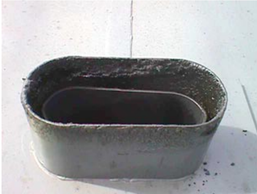
Photograph 5-1. Exhaust Stack with Carbon Build-Up
