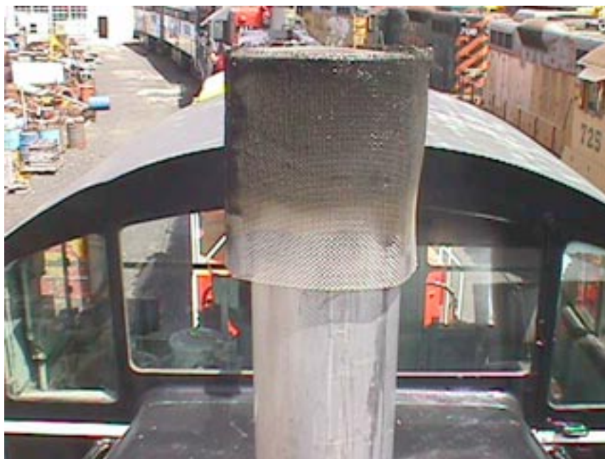
Photograph 5-4. Illegal Screen (Requires an Approved Spark Arrester)
