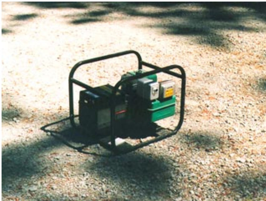
Photograph 5-4. Generator with Spark Arrester and Clearance
