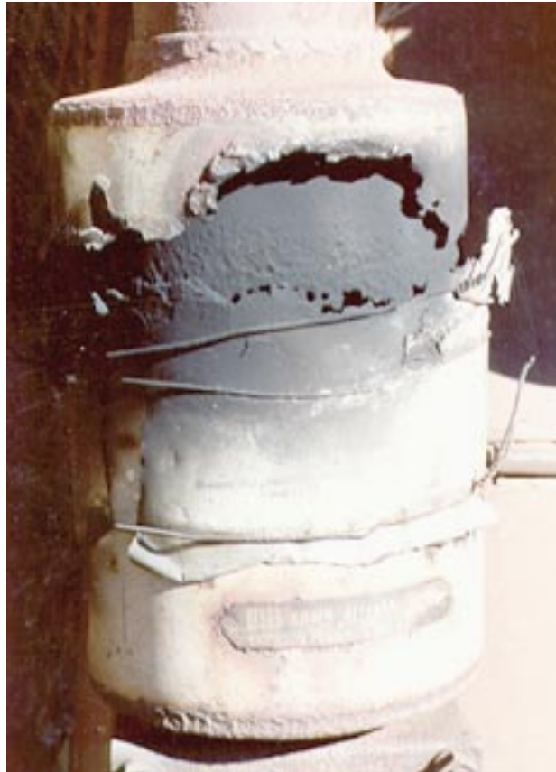
Photograph 9-8. Leaking Exhaust System
