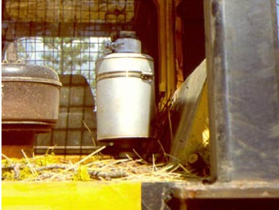
Photograph 4-12. Accumulated Flammables Around Exhaust
