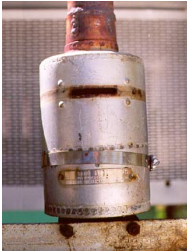
Photograph 4-6. Retention Spark Arrester with Band Removed for Inspection
