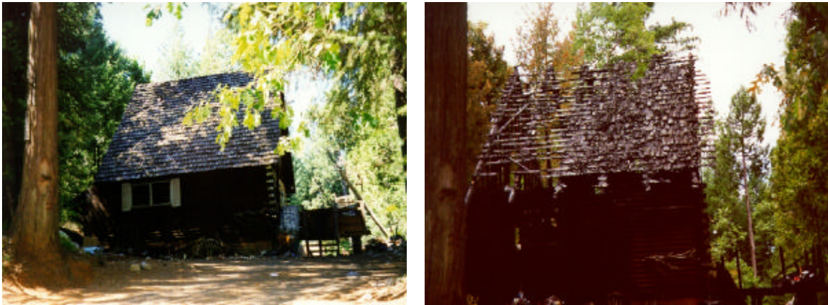
Photograph 9.3. Shake Shingles Before and After a Fire
