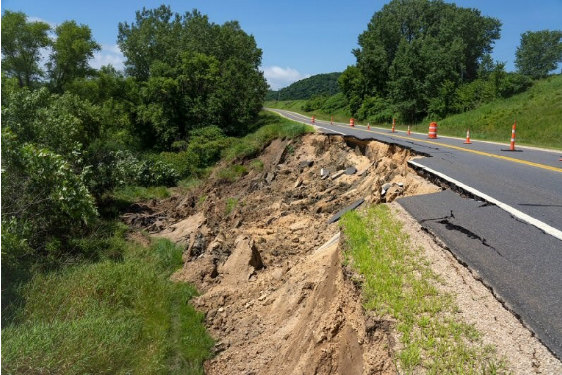
Figure 3.3.2-6: A washed-out road section east of Mount Prairie, WI
