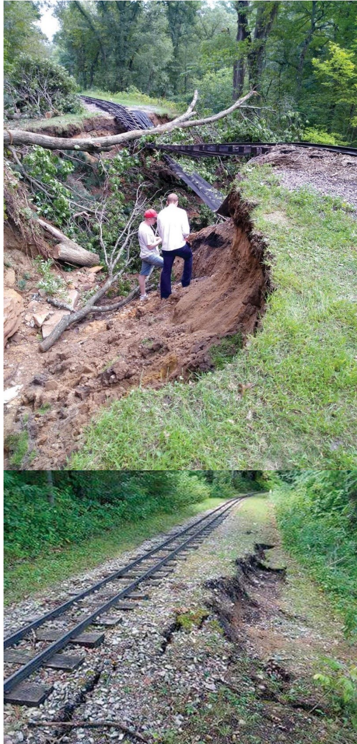
Figure 3.5.2-1: Heavy Rainfall Responsible for Landslides and Erosion that Shutdown the Great Northern Railway in 2018
