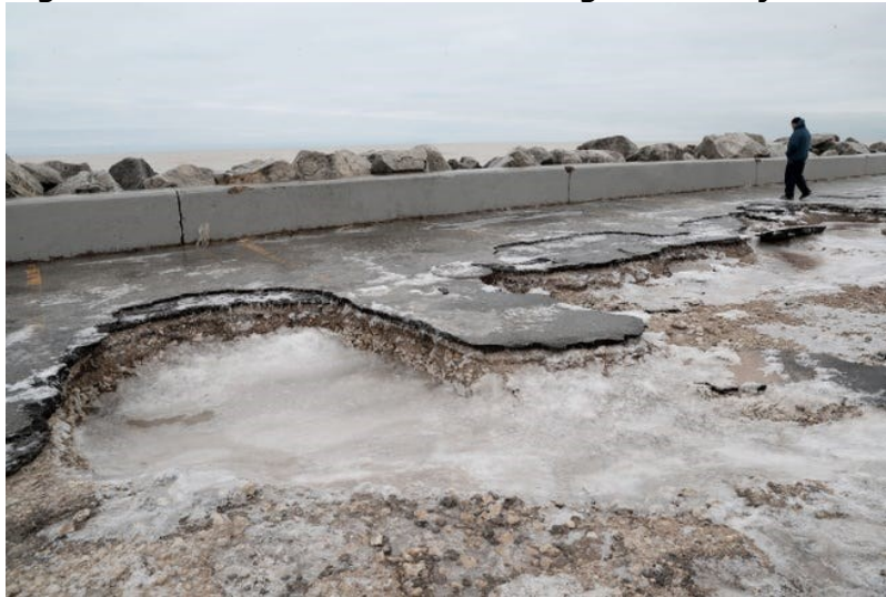
Figure 3.6.2-4: Port Milwaukee Damage, McKinley Marina
