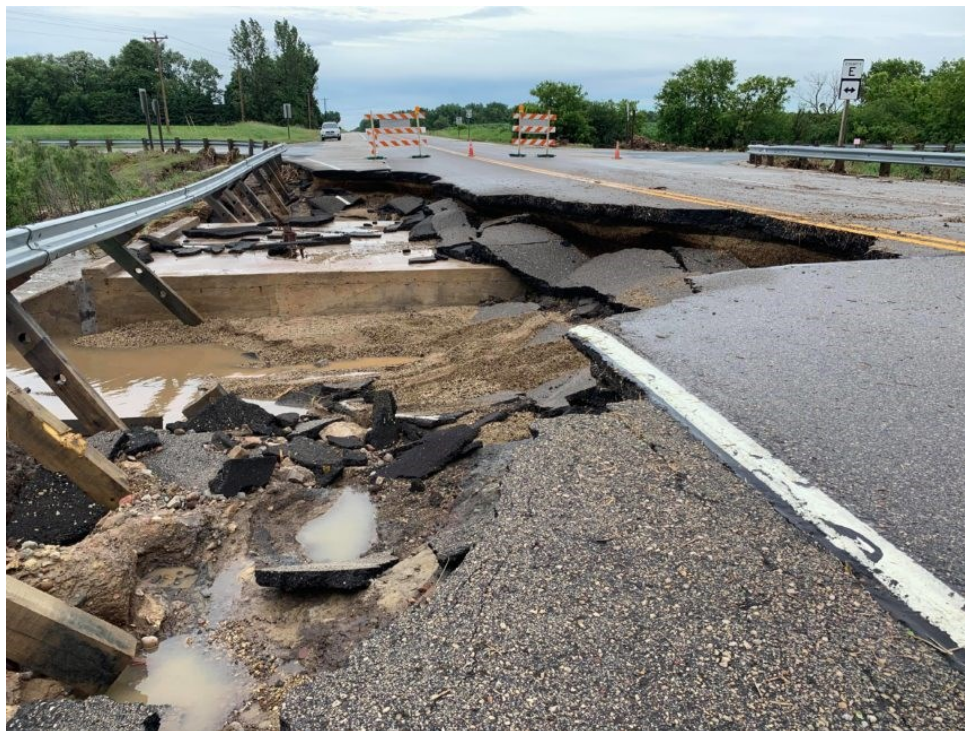
Figure 3.3.2-7: A washed-out road section at the intersection of Highways 63 and E
