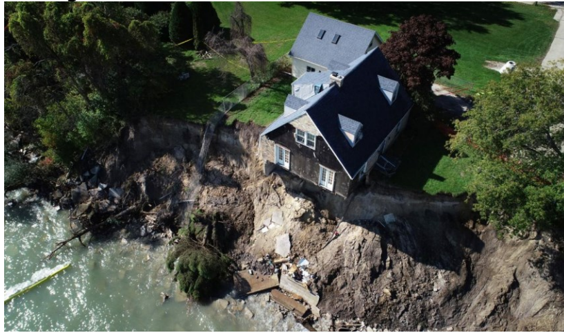
Figure 3.6.2-1: Lakefront Erosion at Somers Home
